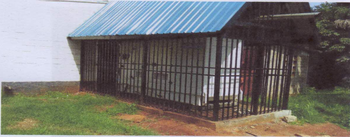
Pic 1.7.2 A generator at Murang'a Referral hospital
