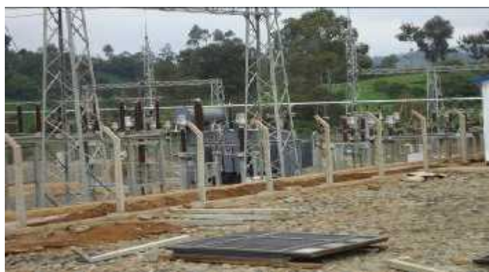
Figure 5: Githambo Power Sub- Station
