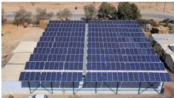
The Arava Solar Plant
