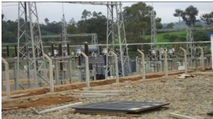
Figure 5: Githambo Power Sub- Station
